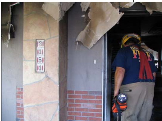
Fire Investigators conducting an investigation after a house fire. They will use their skills and expertise to determine where and how the fire started.
